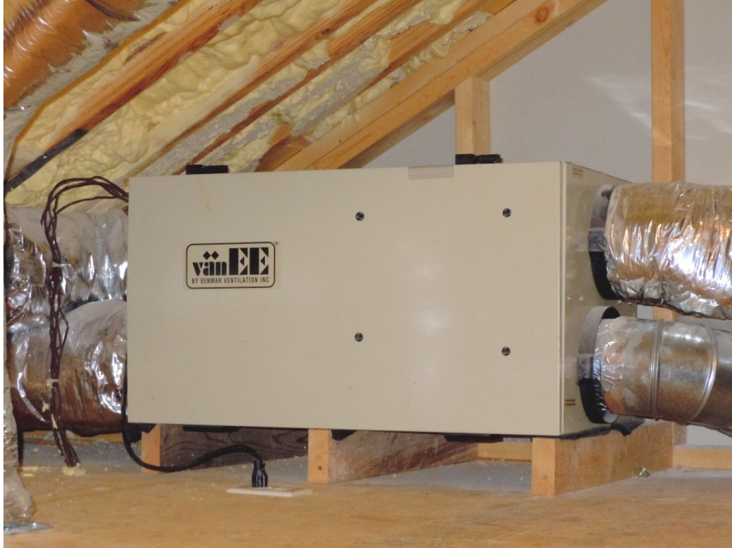
Photograph courtesy of Stitt Energy Systems, Inc., Rogers, Ark.
