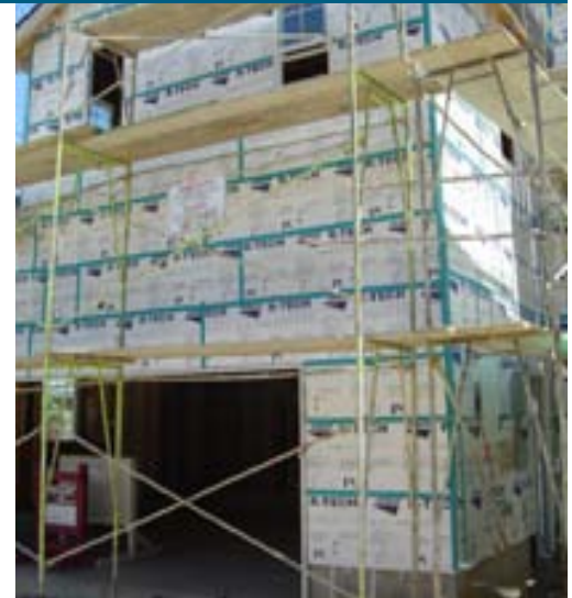
Treasure Homes of Sacramento installs rigid foam under stucco siding to serve as an insulation layer and exterior vapor barrier.
